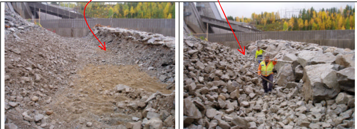
Figure 11 Hällby Dam was in 2004/05 strengthened by a rockfill berm in order to allow for possible large leakages in the future.
